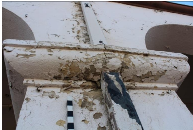
Figure 24. Excess moisture around this downspout on the northwest side of the Depot has caused peeling and loss of paint layers.
