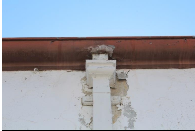
Figure 33. A poor connection between the gutter and downspout has caused water damage to the adjacent paint and stucco.
