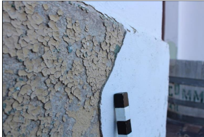
Figure 25. This repair coat of stucco was applied to a column base on the northwest side of the building. Failure to remove deteriorated paint layers prior to application has led to early failure and loss.
