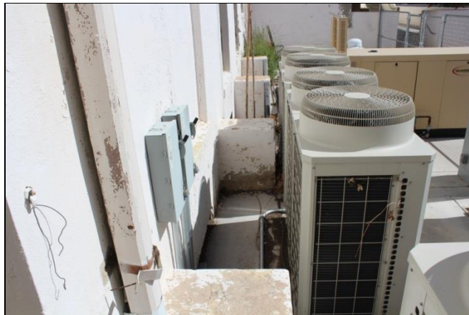
Figure 19. Mechanical equipment on the southeast side of the building may trap water and debris against the foundation and buttresses, and may mask damaging conditions unless this area is regularly inspected.
