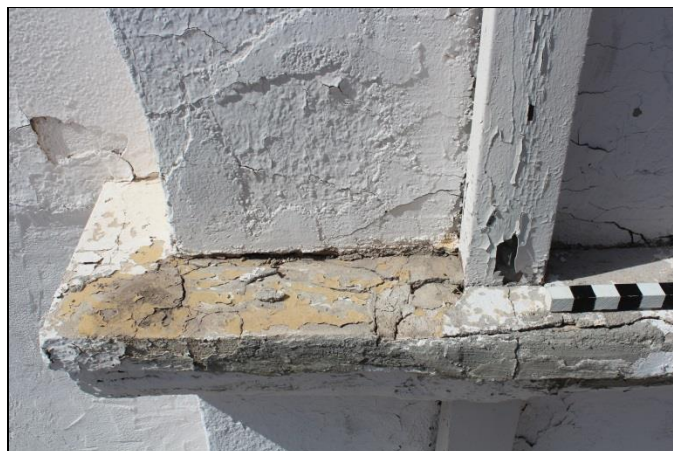
Figure 29. A column capital (NE 05) in poor condition, exhibiting failed repairs, full-depth cracks, and loose materials on the top and sides (Ranking = 4).
