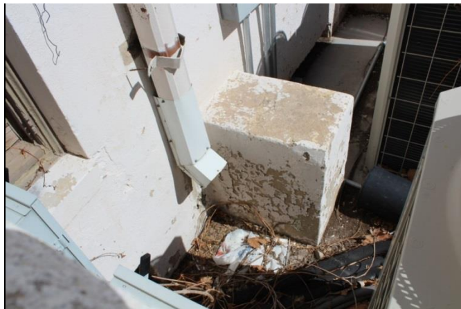
Figure 18. An example of a downspout draining directly against the foundation on the southeast side of the building. All water runoff should be directed away from the building or into an underground collection and dispersal system.
