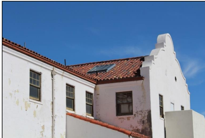
Figure 32. The skylight above the original men's toilet on the southeast side of the building. Failed flashing has resulted in water damage to the interior ceiling.
