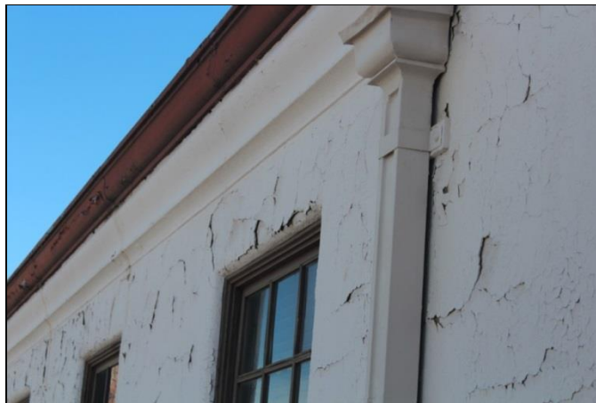
Figure 21. Delaminating stucco at the second floor level on the northwest side of the Depot.
