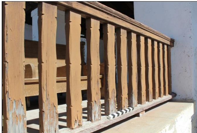
Figure 40. An intact wood railing spanning between columns of the pergola. Note the notched and beveled balusters.
