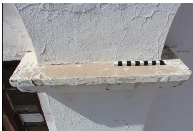
Figure 26. A column capital (NE 04) in very good condition, exhibiting few cracks or repairs (Ranking = 1).
