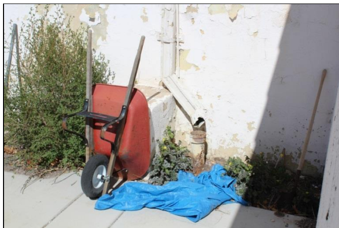
Figure 35. A failed connection between a downspout and drain on the southeast side of the building. The location and condition of the drain field is unknown.
