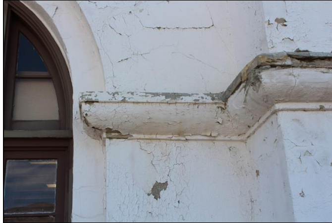
Figure 23. Failure to remove deteriorated paint layers prior to the application of new paint has led to cracking, alligating, blistering, detachment, and full loss of paint layers.
