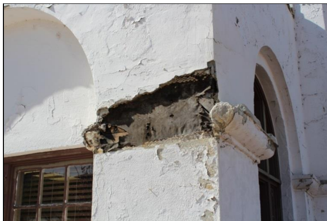
Figure 30. A column capital (NW 01) in very poor condition, exhibiting complete loss and exposing the building paper and wooden sheathing and blocking (Ranking = 5).
