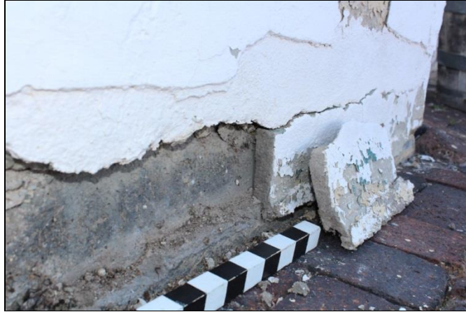
Figure 16. Detail of poured concrete foundation on northwest wall where overlying stucco layer has failed. Note absence of building paper and metal lath.
