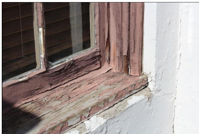
Figure 37. Failed paint layers and cracked, weathered wood are common on window sills and the bottom rails of window sashes.
