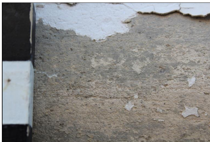
Figure 13. Original appearance of finish coat used for column capitals. Note the lack of visible aggregate and smooth finish. Scale is marked in 1-inch increments.
