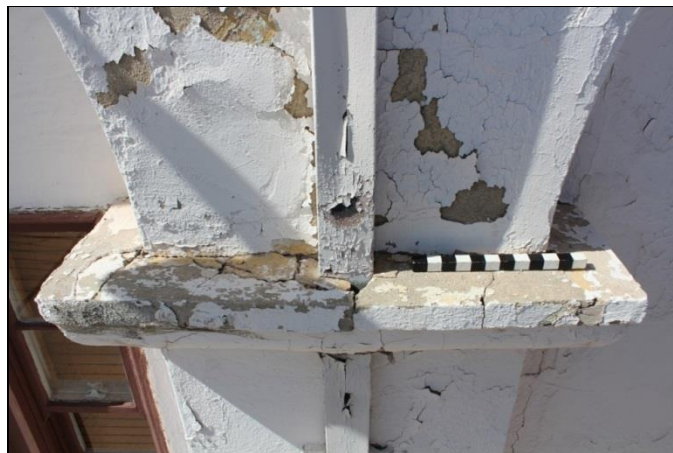
Figure 28. A column capital (NE 02) in fair condition, exhibiting repairs, full-depth cracks, and loose materials on the top side (Ranking = 3).
