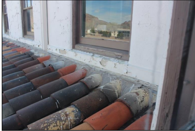
Figure 31. Original (dark) and replacement (red-orange) roof tiles over the arcade on the northwest side of the Depot. The flashing between the tiles and the wall is aged but generally in good condition.
