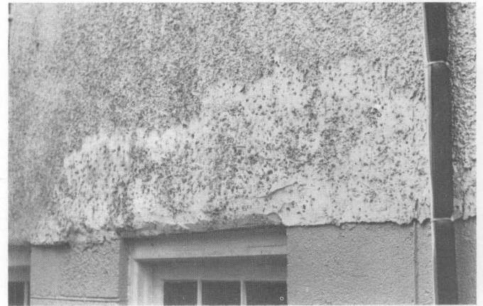
Fig. 14. This poorly executed patch is not the work of a professional plasterer. While it may serve to keep out water, it does not match the original surface, and is not an appropriate repair for historic stucco. Photo: Betsy Chittenden.
