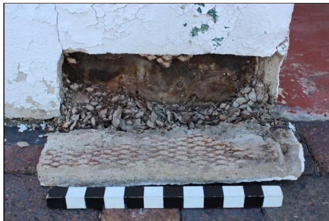
Figure 14. Stucco sample taken from the base of Column NW 06 on the northwest façade, central arcade. Scale is marked in 1-inch increments.
