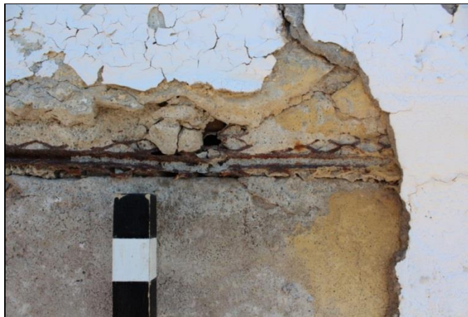
Figure 22. Exposed and corroded lath at the base of a column on the pergola.
