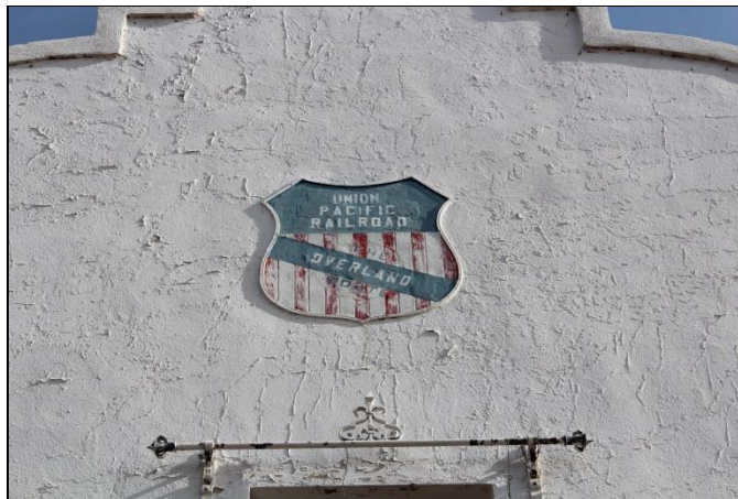
Figure 20. Hairline cracks in the stucco that have telegraphed into overlying paint layers.
