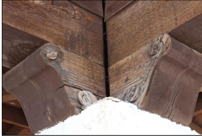
Figure 39. Decorative wood scrollwork (detached on the right and missing on the left), which was applied to the scrolled brackets supporting the pergola roof.
