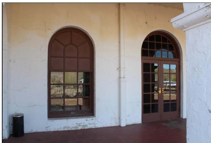
Figure 36. Windows and doors protected by arcades are in very good condition, despite minor alterations like painted glazing.
